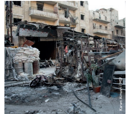
The airstrikes shattered everything in the surrounding area, including ambulances and cars parked in the front of the hospital.
