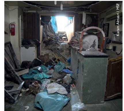
The hospital's main reception area was shattered by the bombing.
