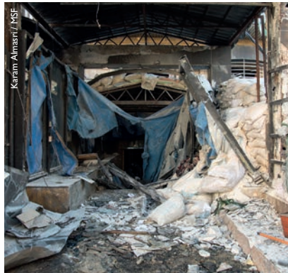
The main entrance of the hospital after it was bombed
